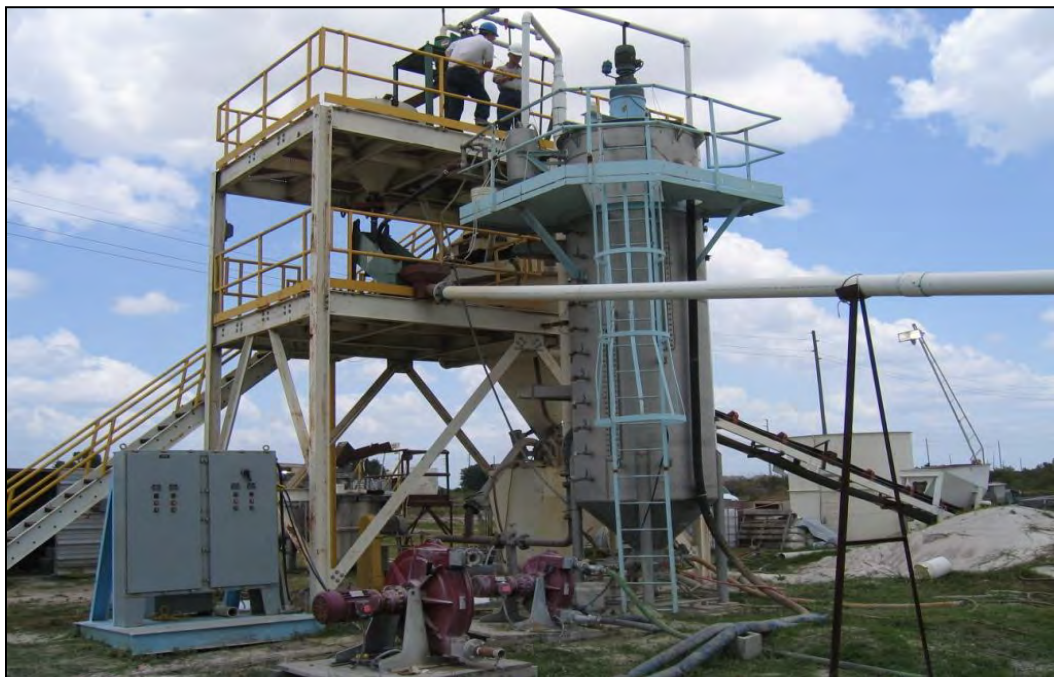
Pilot plant for the FIPR Institute's Deep Cone™ paste technology.
