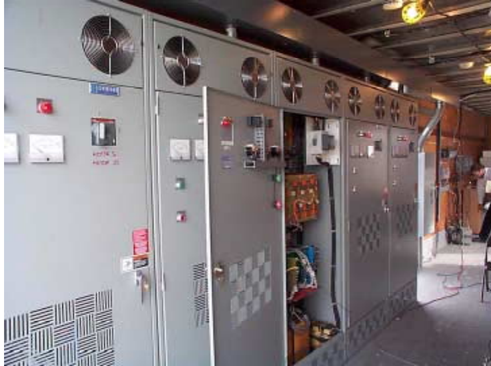
Figure 10. Five 100 HP Motor Control Units Shared Between Ten Motors.
