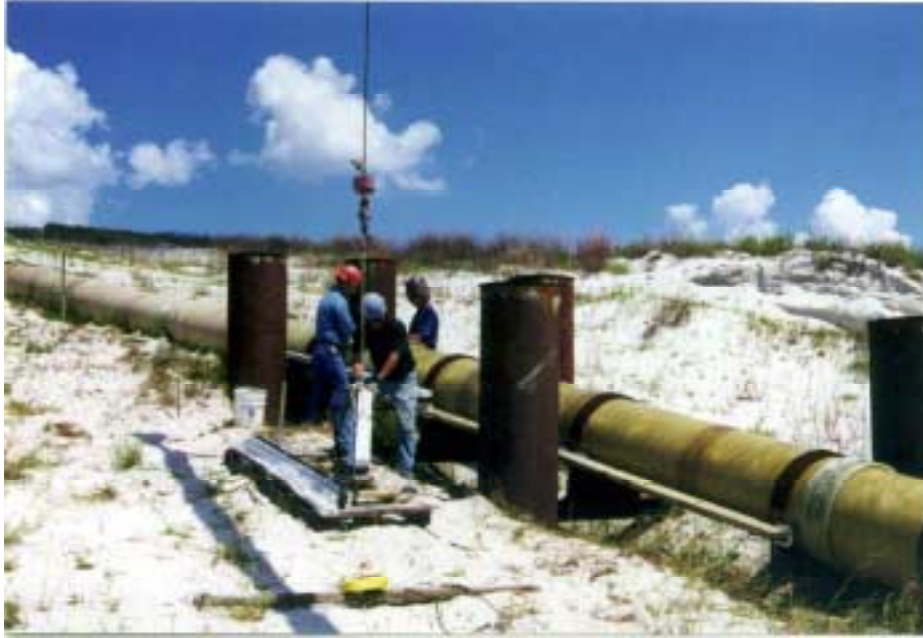
Figure 8. Switch Demonstration Magnets in the Process of Installation on the 30-Foot Long, 200-Foot Radius Horizontal Curve.
