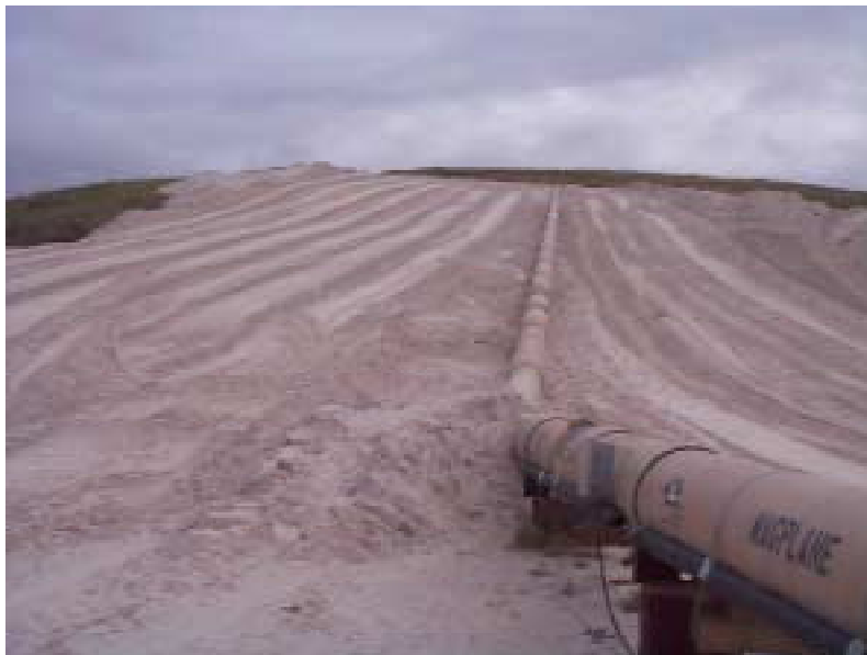
Figure 5. Lakeland Demonstration Project Hill Climb. Motors Number 9 and 10 Are Shown in the Foreground.
