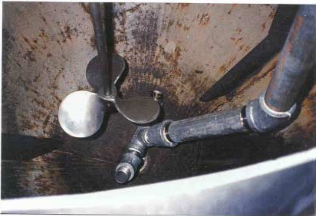
Figure 10. Feed Sump with Slurry Feed Control Valve and Pulp Circulation System.
