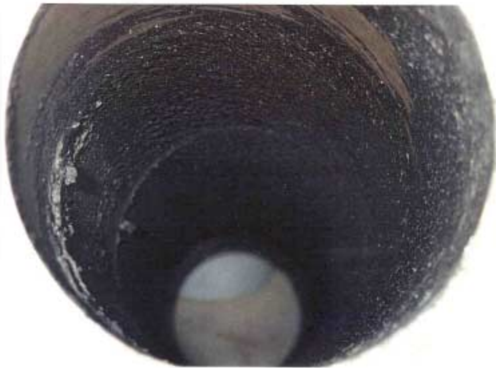
Figure 42. Crud Deposit on the Surface of the Porous Tube.
