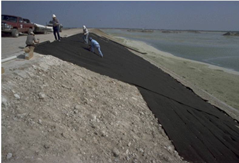
Figure 6. Installation of Additional Geofabric on Northern Geodrain Test Section. Apr 06, 1999; t = -20 days; Pond Level = 124.4 ft msl [04/14/99: 3]
