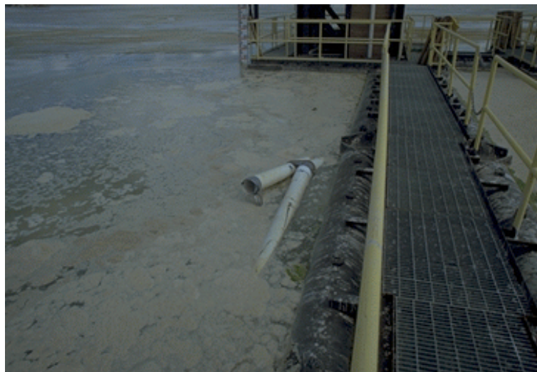
Figure 18. Lateral Pipelines Pulled Apart at Joints. Nov 19, 1999; t = +207 days; Pond Level = 132.5 ft msl [12/16/99: 20]
