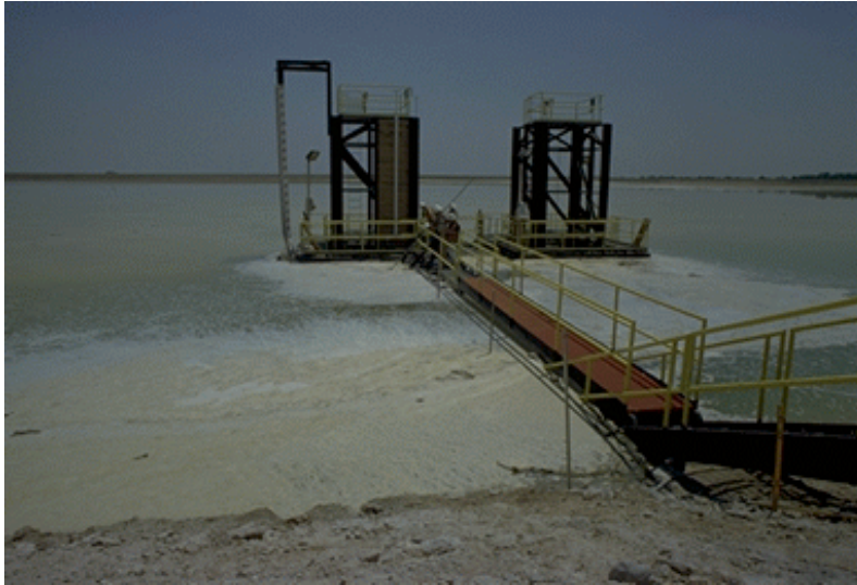
Figure 14(a). Installation of Steel Pipe Piles for Support of Lateral Pipelines. Apr 20, 1999; t = -6 days; Pond Level = 125.6 [04/28/99: 31]
