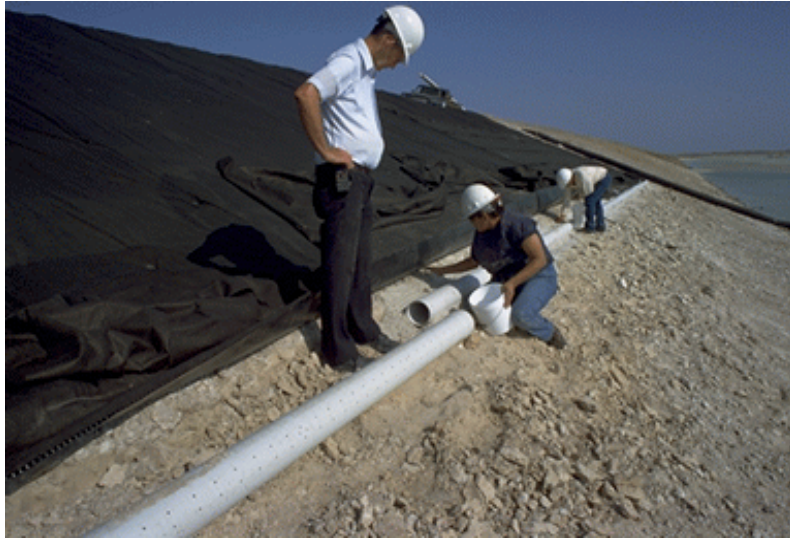
Figure 7(a). Installation of Toe Drain for Northern Geodrain Test Section. Apr 07, 1999; t = -19 days; Pond Level = 124.4 ft msl [04/14/99: 15]
