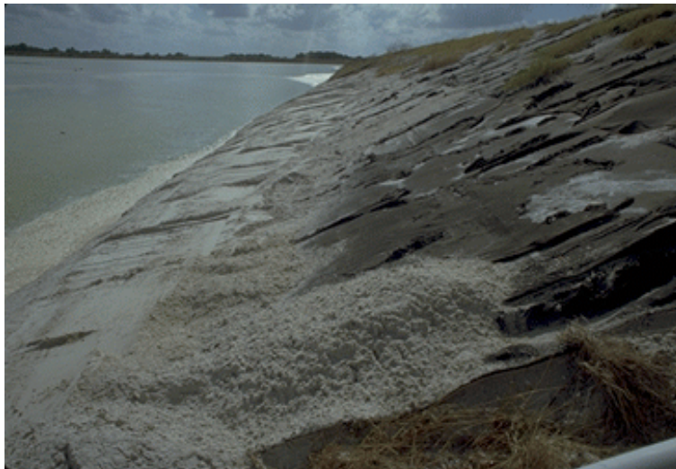
Figure 10. Southern Geodrain Test Section: Additional Tailings Sand Placed on Toe Drain (Second Time). Nov 19, 1999; t = +207 days; Pond Level = 132.5 ft msl [12/16/99: 23]
