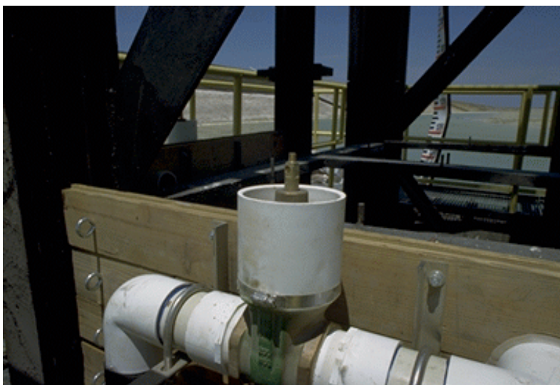
Figure 17(b). PVC-Brass Valve Assembly for Southern Geodrain Test Section Mounted on Spillway.
