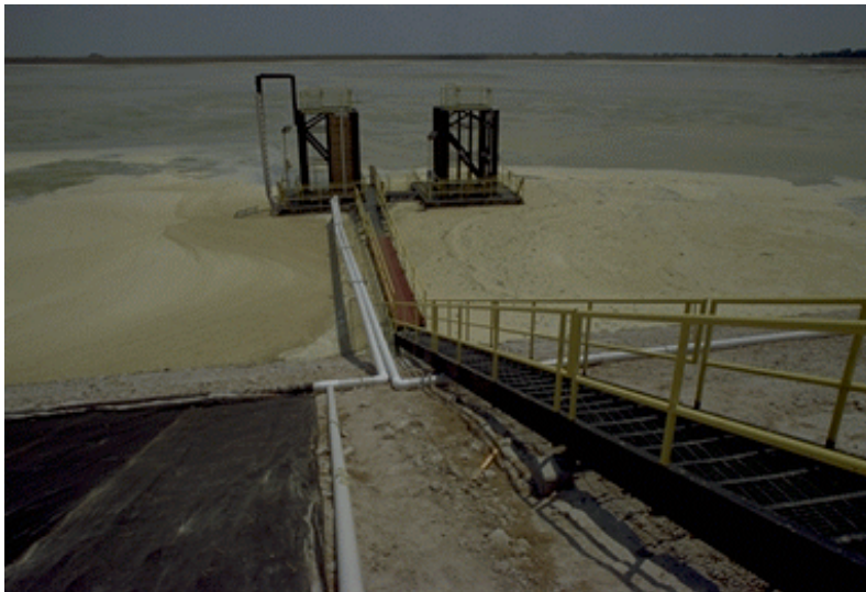
Figure 14(b). Installation of Steel Pipe Piles for Support of Lateral Pipelines. Apr 26, 1999; t = 0 days; Pond Level = 125.8 ft msl [06/08/99: 9]
