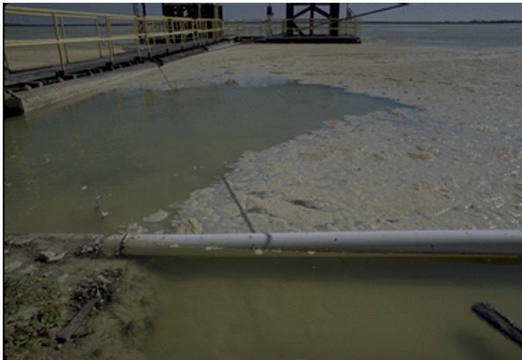
Figure 13. Longitudinal Conveyance Pipeline Floating Free from Anchors. Feb 16, 2000; t = +296 days; Pond Level = 134.5 ft msl [03/15/00: 15]
