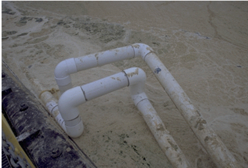
Figure 19. Repaired Elbows at Lateral Pipeline Joints. Nov 24, 1999; t = +212 days; Pond Level = 132.5 ft msl [12/27/99: 7]
