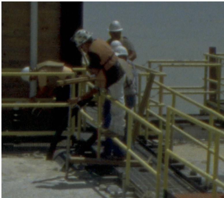
Figure 15(a). Installation of Flexible Hoses Connecting Lateral Pipelines to Spillway. Apr 20, 1999; t = -6 days; Pond Level = 125.6 ft msl [04/28/99: 34 (enlargement)]
