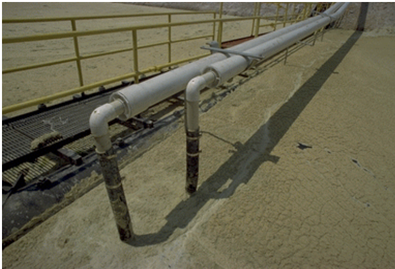
Figure 15(b). Installation of Flexible Hoses Connecting Lateral Pipelines to Spillway. Apr 26, 1999; t = 0 days; Pond Level = 125.8 ft msl [06/08/99: 11]
