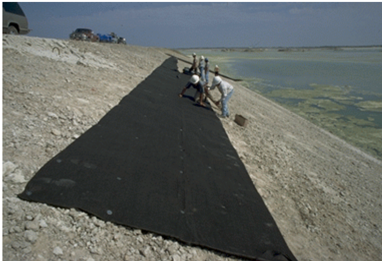
Figure 2. Installation of Northern Geodrain Test Section. Apr 05, 1999; t = -21 days; Pond Level = 124.1 ft msl [04/12/99: 34]
