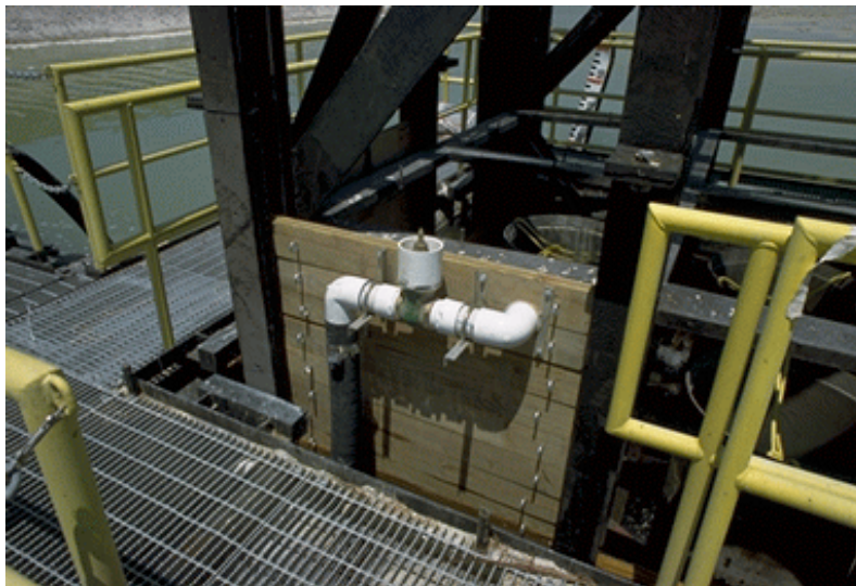
Figure 17(a). PVC-Brass Valve Assembly for Southern Geodrain Test Section Mounted on Spillway.
