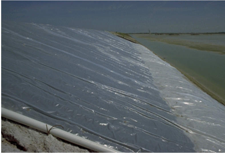
Figure 9. Northern Geodrain Test Section: Additional Tailings Sand Placed on Toe Drain and Entire System Covered with Polyethylene Plastic Sheet. May 28, 1999; t = +32 days; Pond Level = 127.7 ft msl [06/21/99: 11]
