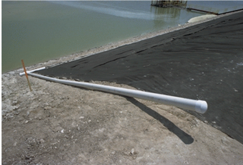
Figure 11(a). Standpipe N-1 at North End of Northern Geodrain Test Section. Apr 07, 1999; t = -19 days; Pond Level = 124.4 ft msl [04/14/99: 27]
