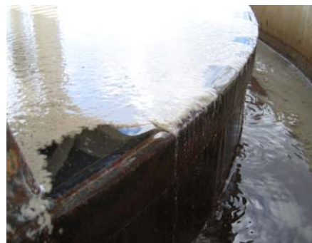
Figure 6. The Clarifier Under Improper Running Conditions.
