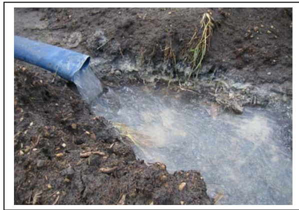
Clear Water Coming Off the Clarifier During a Smooth Run
