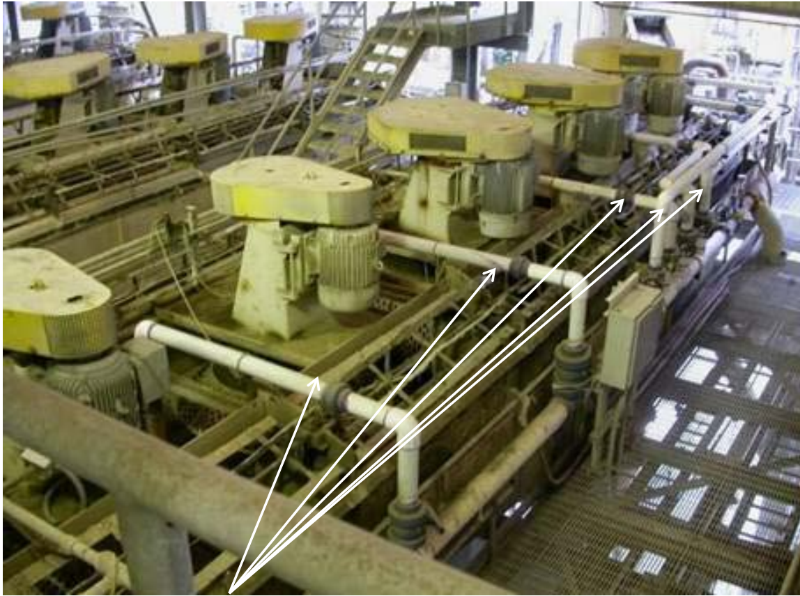
Picobubble slurry distribution pipes
