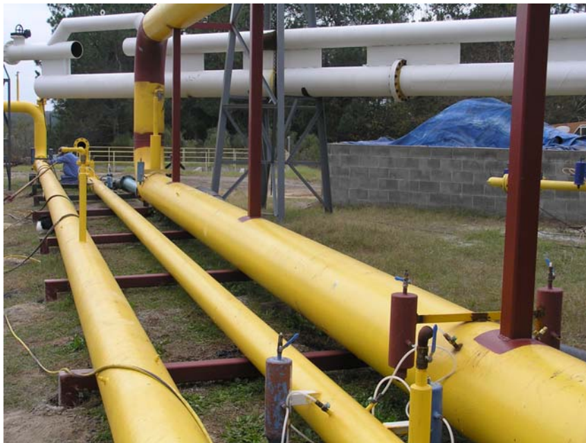
Figure D-6. Orifice Plate and 35 Ft. Horizontal Loss Section.
