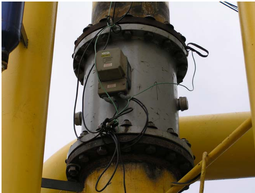
Figure D-4. Pressure Transducers and Magnetic Flowmeter.
