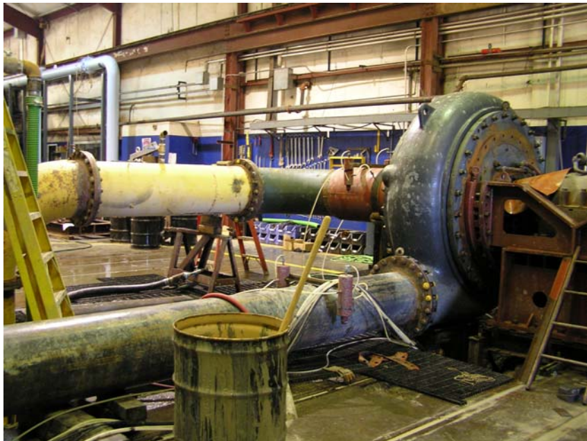
Figure D-2. Pump Suction and Discharge Pipe.
