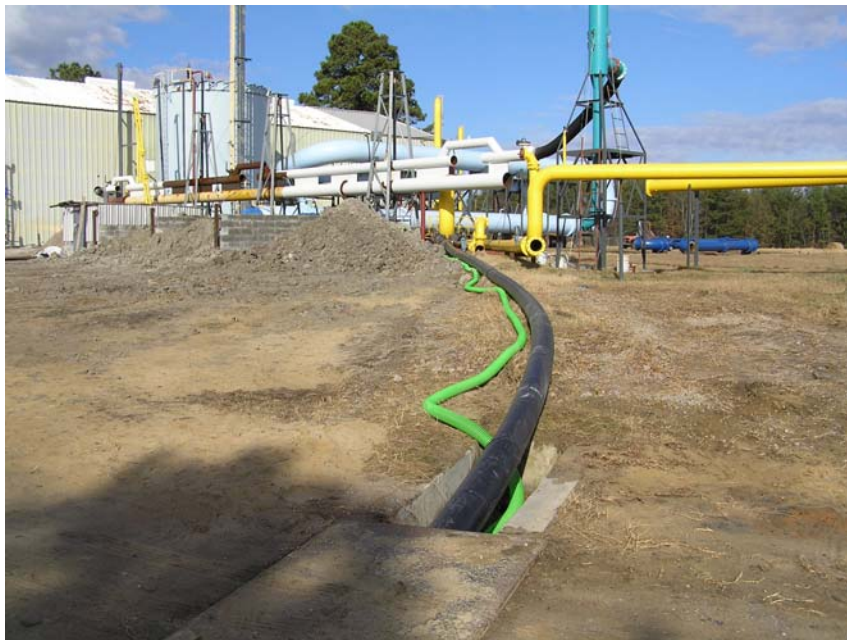
Figure D-8. 8" Flush Valves and 8" Flush HDPE Pipeline.
