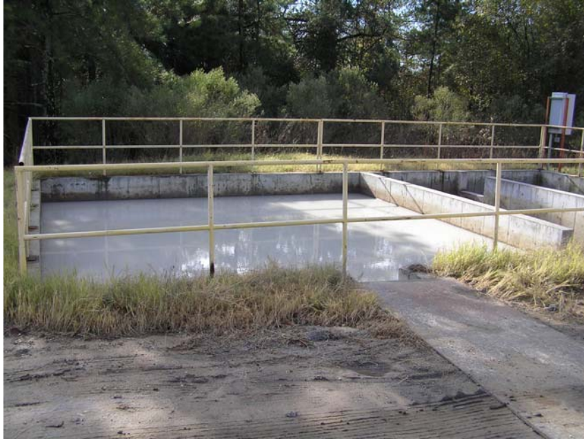
Figure D-9. Slurry Disposal Collection Pond.
