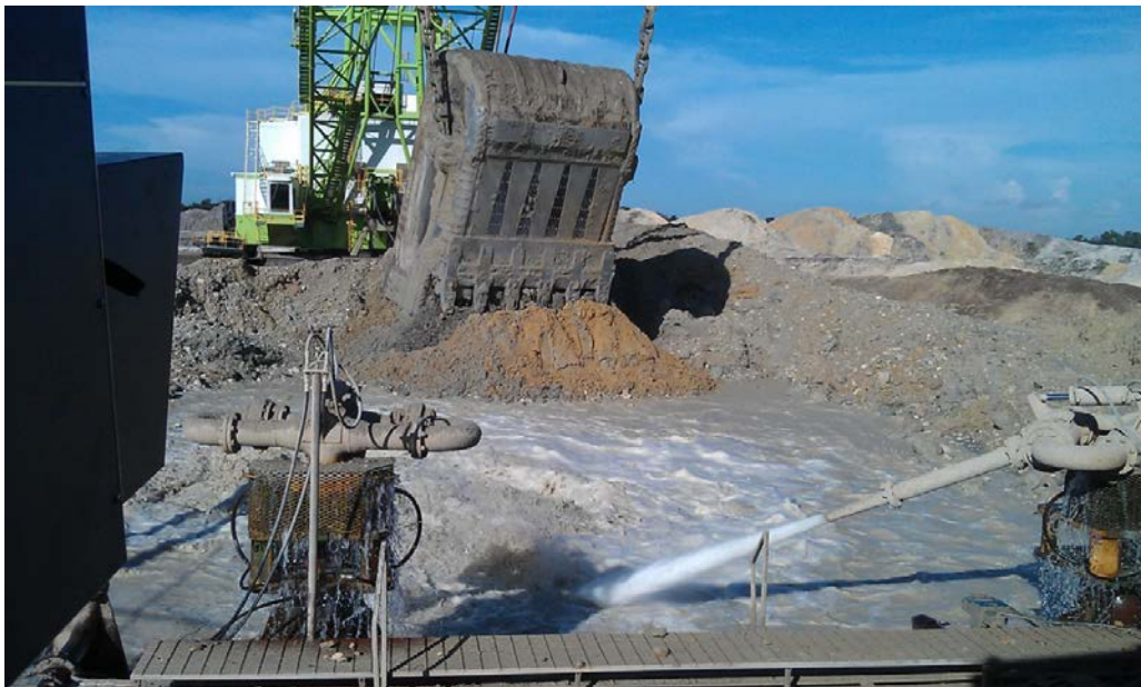
Figure 19. ReLIBS Unit Situated at the Washing Pit Site Facing Matrix Rock Delivered by the Dragline.
