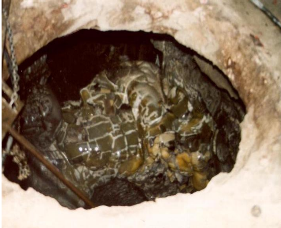
Figure 11. Scale Build-up in a Phosphoric Acid Attack Tank
