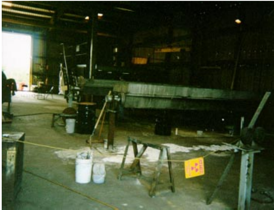
Figure 39. Filter Pan Repair Area - Open on Both Sides
