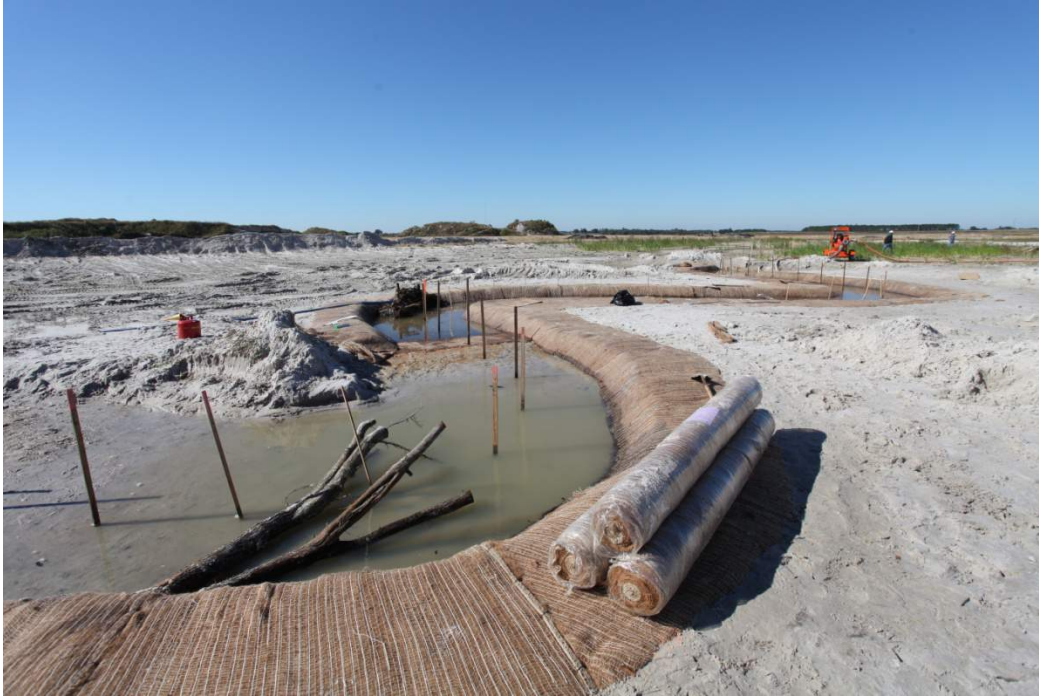
B) Channel excavated from the floodplain and banks wrapped in erosion control blanket.
