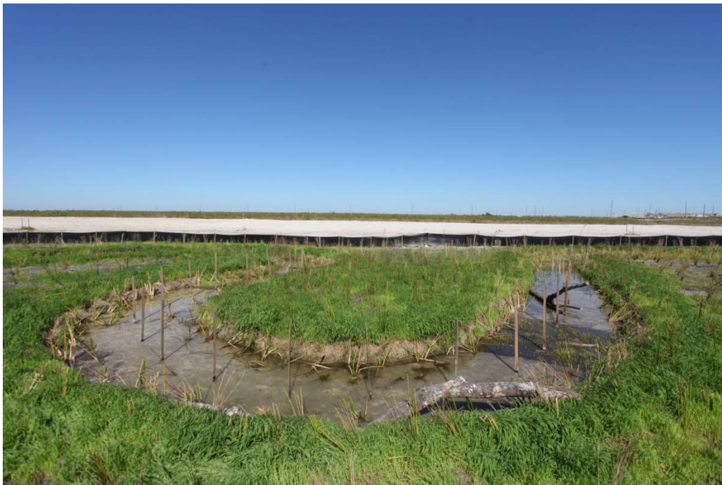
C) Works stabilized with temporary groundcover prior to planting permanent cover. North Gilshey Branch, Fort Meade Mine
