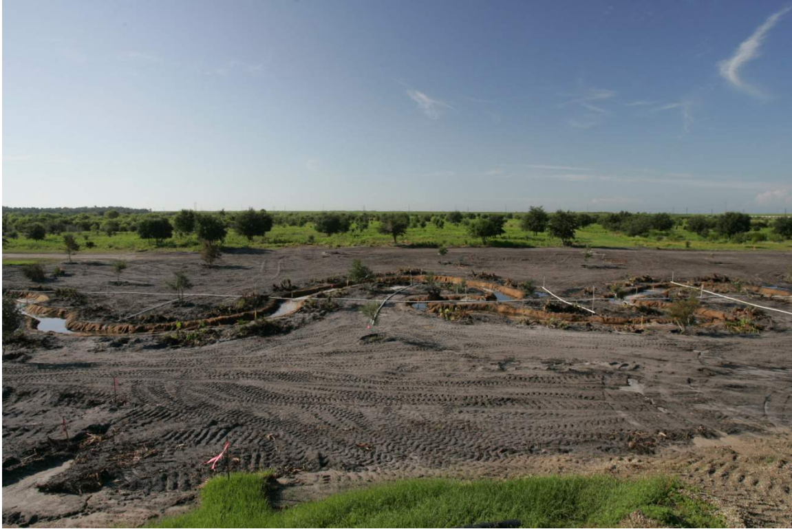
E) Project overview upon earthwork completion, prior to installing vegetation. DB-5, South Pasture Mine
