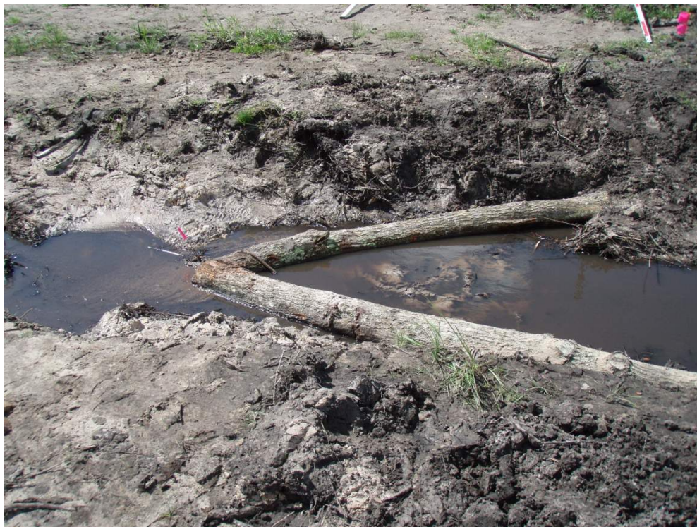
C) V-log weir placed after 4 weeks of hydraulic carving to induce a new pool.
